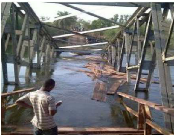
Mabang bridge collapse
