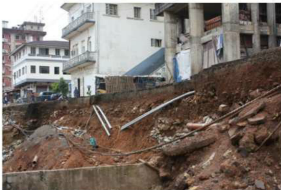
Recent landslide at King Jimmy resulting from bridge failure
